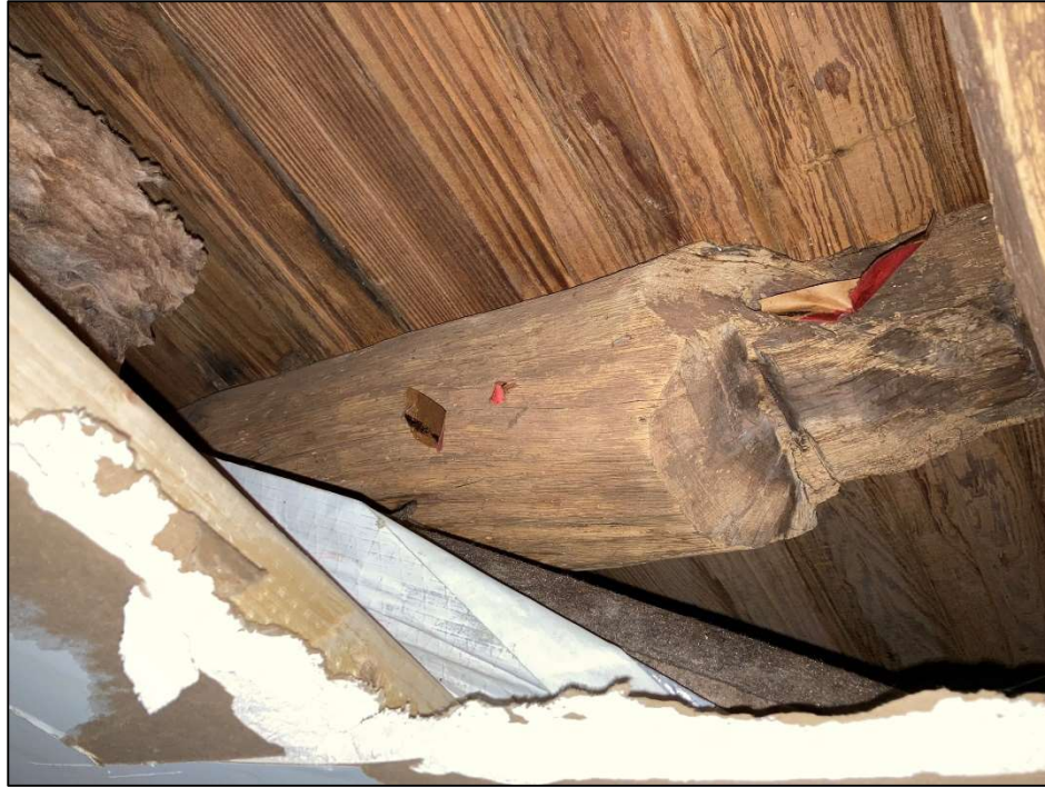
Figure 41. Basement, below enclosed side porch. Looking the other way through the same hole shown in the previous photo. This hewn joist is notched into the beam shown in the previous photo and supports the enclosed side porch. May 2023. Photo by the author.
