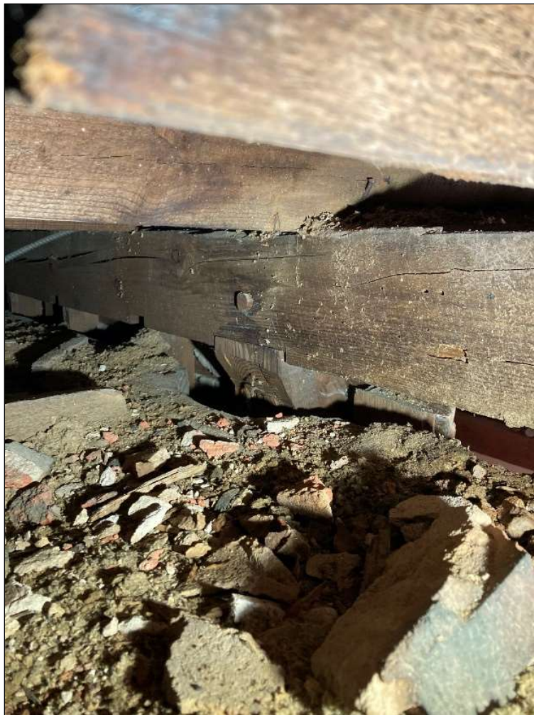
Figure 64. Attic, above log section looking at frame construction of the front frame section of the house. Horizontal beam is the top plate in the frame wall, notice the vertical beams mortised and pegged into it. May 2023. Photo by the author.
