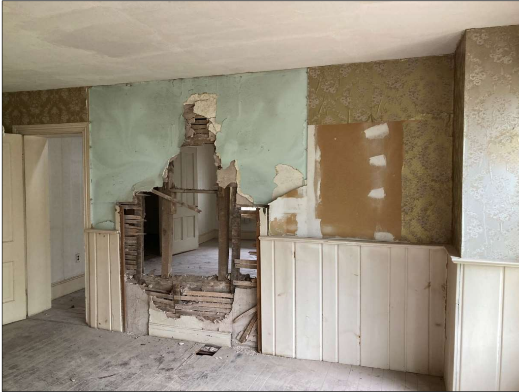
Figure 31. First floor, dining room (log section), looking at wall between log and frame sections. May 2023. Photo by the author.
