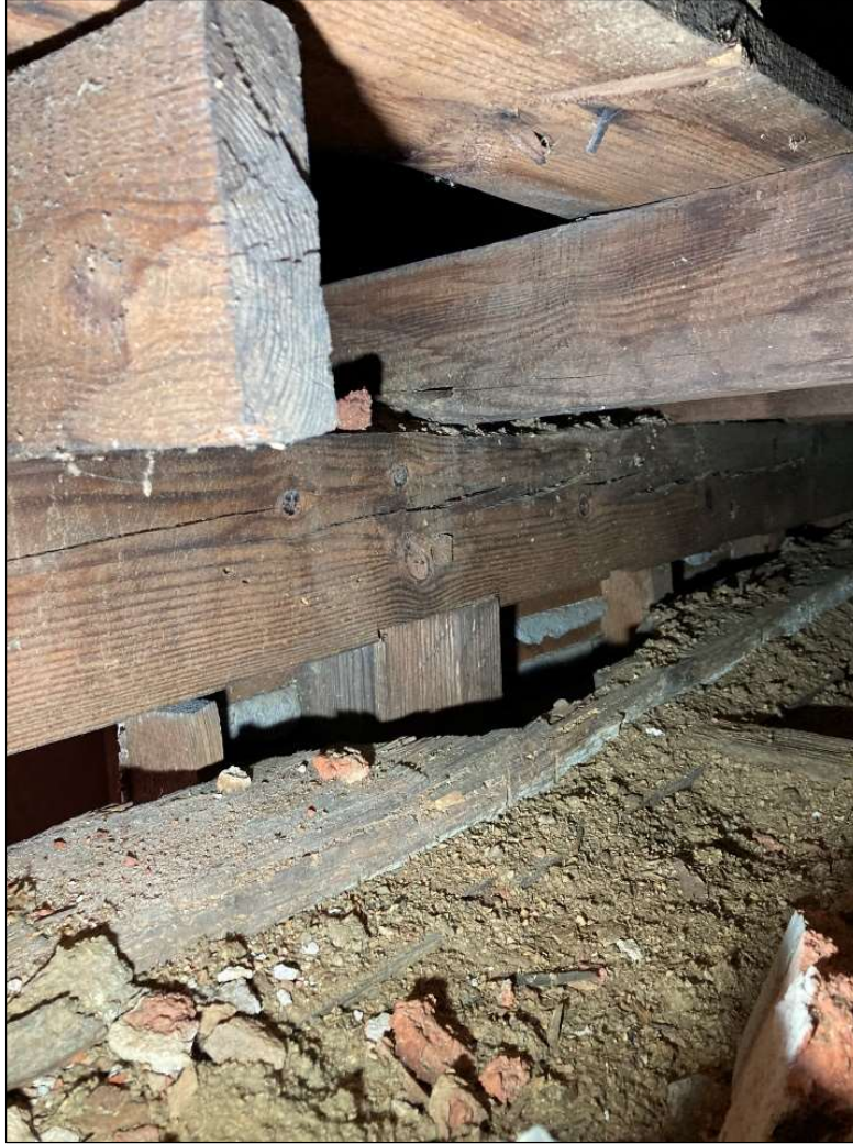
Figure 65. Attic, above log section looking at frame construction of the front frame section of the house. The horizontal beam in the center of the photo is the top plate of the frame section of the house, with vertical members mortised and pegged into it below. Just below that plate in the photo is the top log in the log wall that abuts the frame section of the house. Notice that this log has the remains of whitewash on one side, suggesting it is probably reused in this location. May 2023. Photo by the author.
