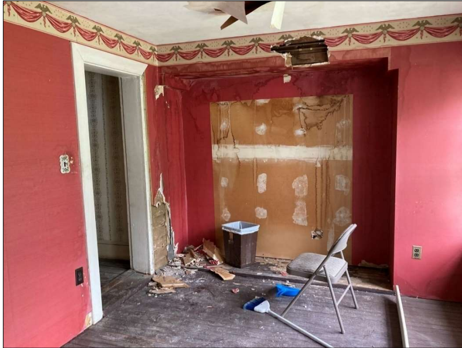
Figure 35. First floor, enclosed side porch, looking at rear wall and doorway connecting to rear hall in log section. Area of exposed weatherboard siding is shown beside the doorway. May 2023. Photo by the author.
