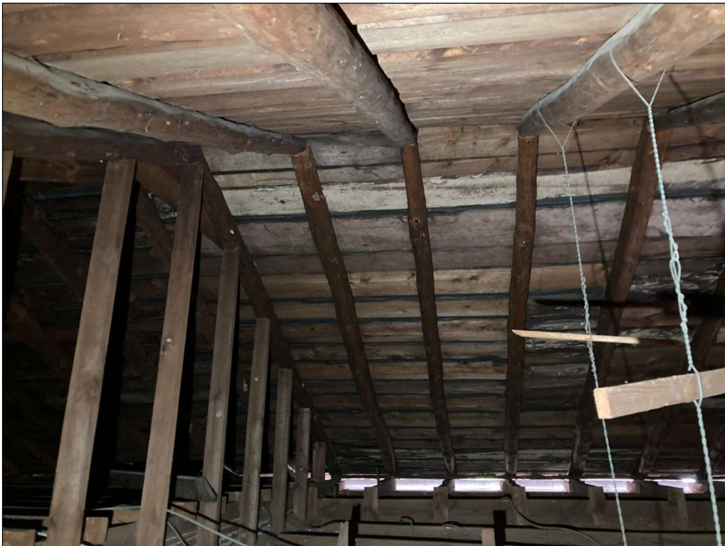
Figure 63. Attic above log section, looking up at ridge. May 2023. Photo by the author.
