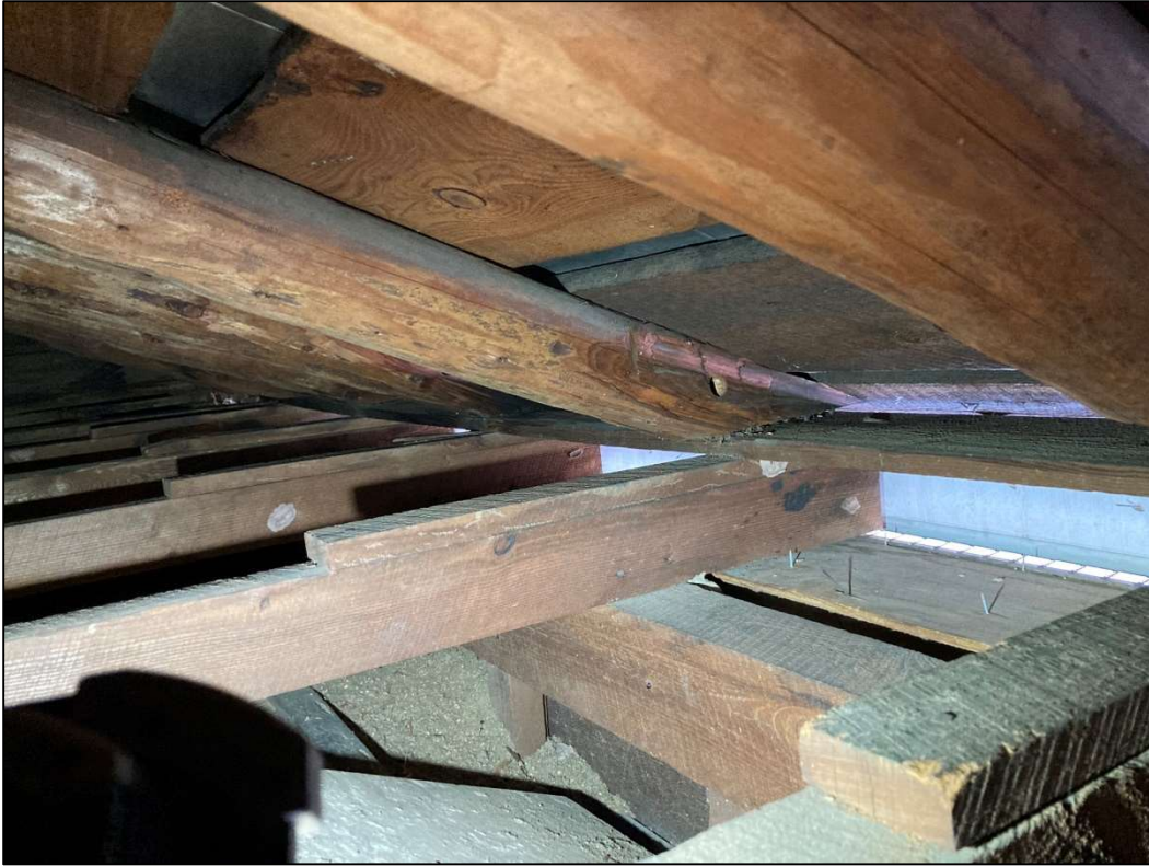
Figure 62. Attic above log section, looking at board false plate and rafter ends. May 2023. Photo by the author.
