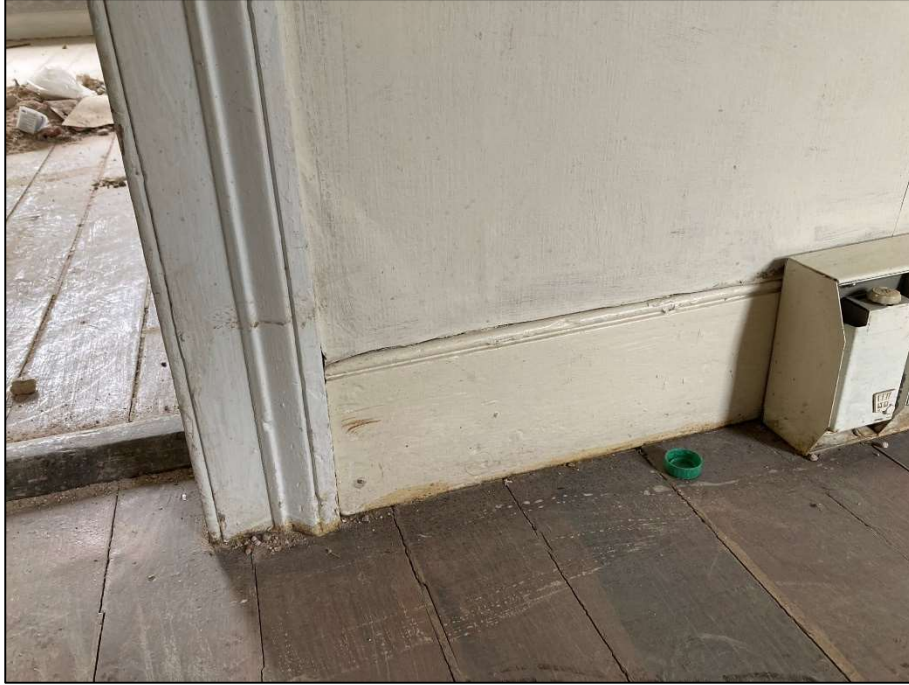
Figure 44. Second floor, rear hall, detail of baseboard and door trim on partition wall in log section. May 2023. Photo by the author.
