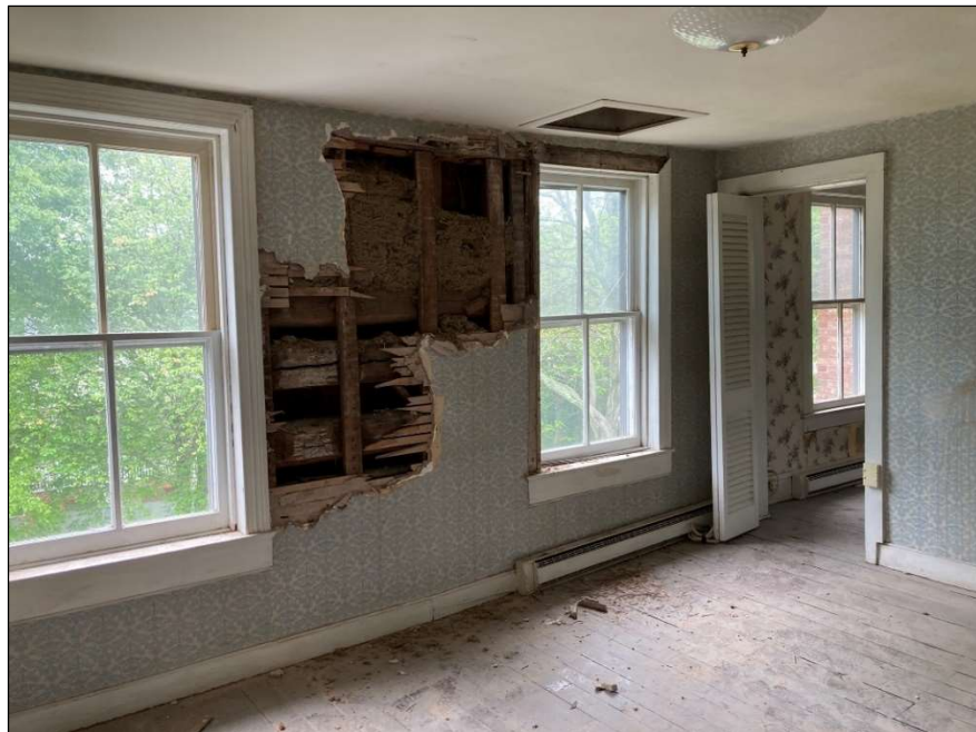
Figure 50. Second floor, bedroom above dining room (log section), looking at east (exterior) wall and doorway to the rear addition. May 2023. Photo by the author.
