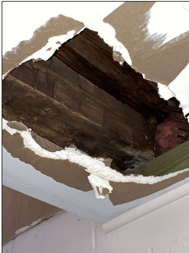
Figure 40. Basement, below the enclosed side porch. This hole in the drywall is the only place where the framing of the house is visible from below. This heavy, hewn beam supports the enclosed side porch. May 2023. Photo by the author.
