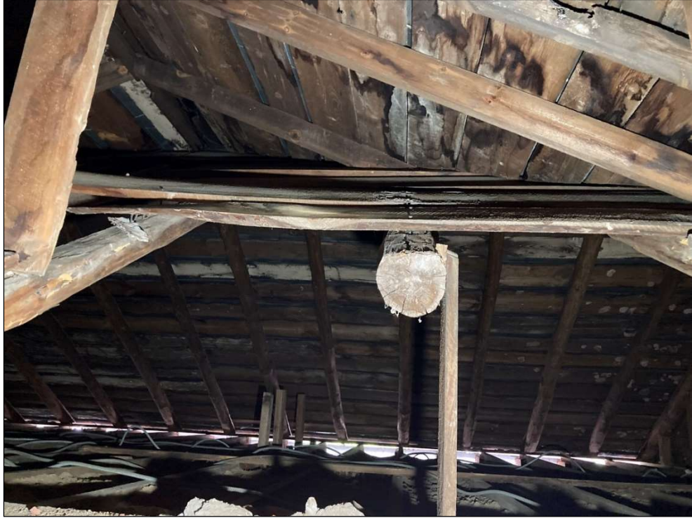
Figure 66. Looking through the hole where the chimney used to be at the roof construction of the frame section of the house. May 2023. Photo by the author.
