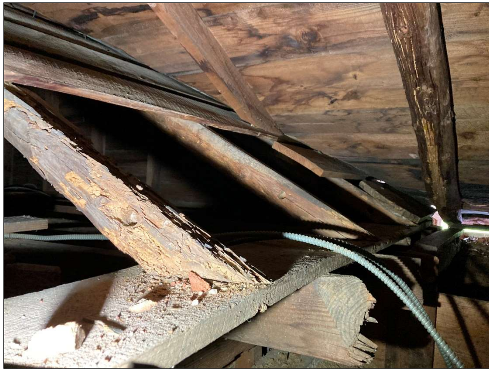
Figure 67. Attic, looking at the rear slope of the roof of the frame section of the house and the later roof that encloses it. Horizontal board is a board false plate supporting the ends of the pole rafters. May 2023. Photo by the author.
