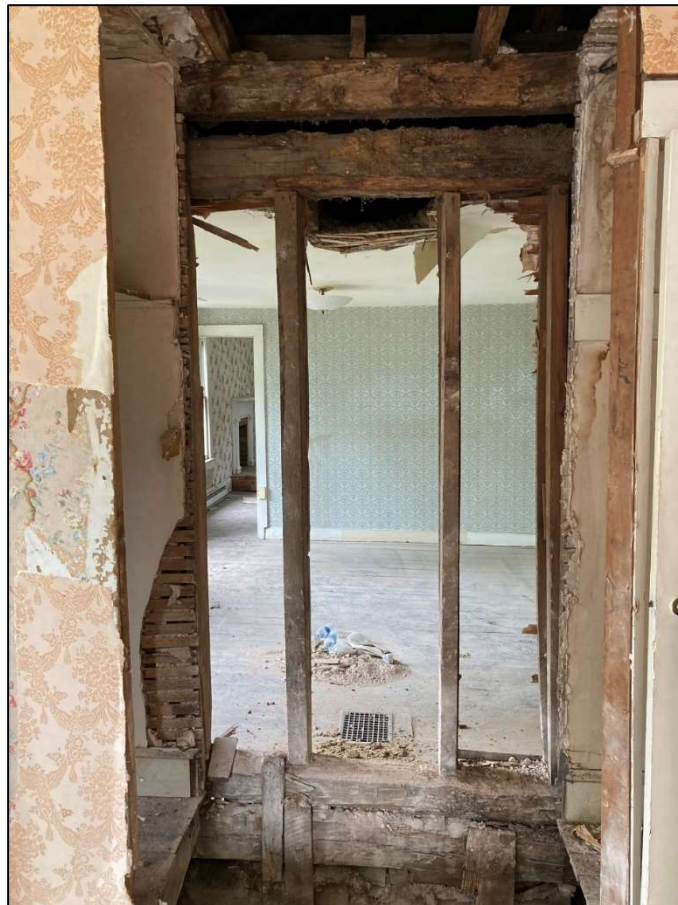
Figure 48. Second floor, looking through the wall where the stone chimney used to be from frame section into log section. May 2023. Photo by the author.
