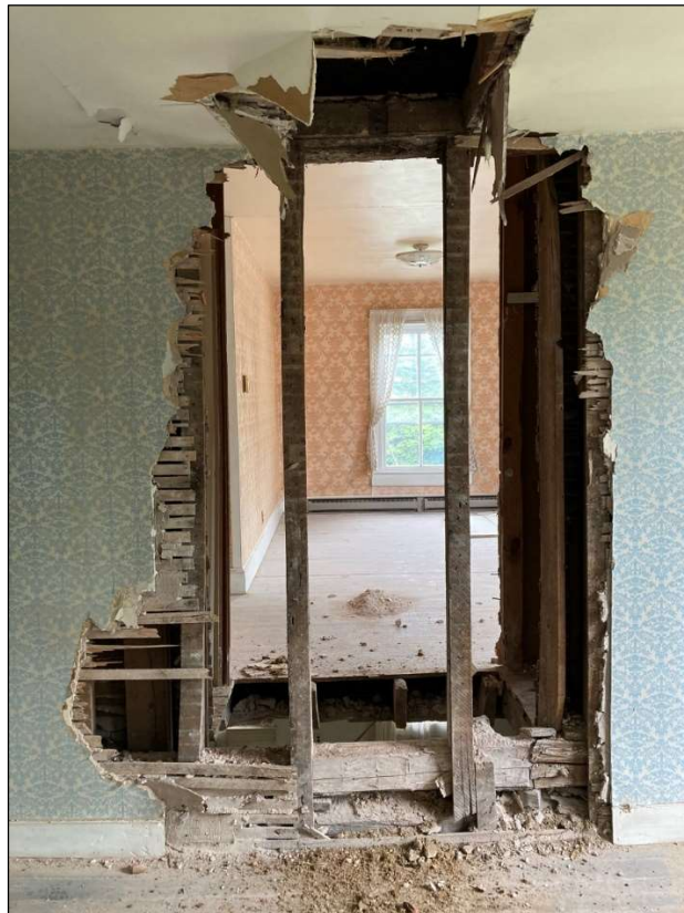
Figure 46. Second floor, bedroom above dining room (log section), looking at the wall between log and frame sections where the chimney was removed. May 2023. Photo by the author.
