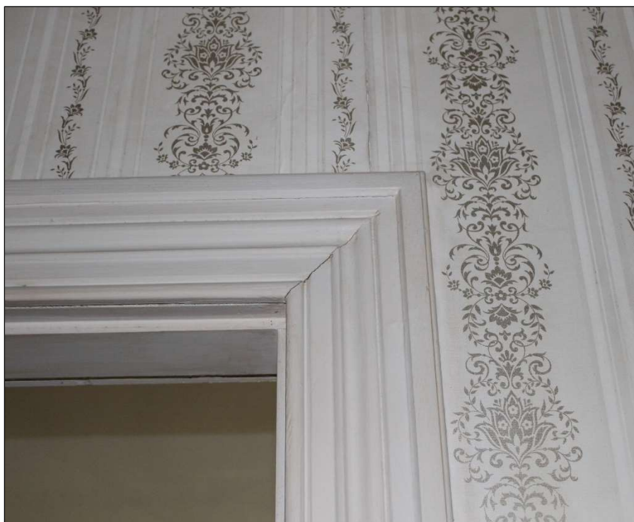
Figure 22. First floor, door trim in front hall. May 2023. Photo by the author.
