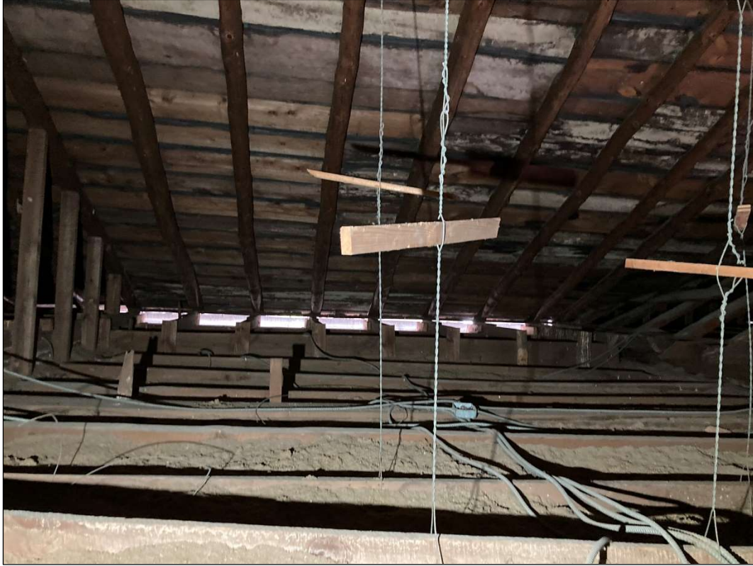
Figure 61. Attic, above log section, looking west from hatch near east wall. Note the joists running north south (across the picture in the foreground) and the roof rafters running east-west. The outriggers constructed to carry the ends of the rafters are visible towards the middle of the image. May 2023. Photo by the author.
