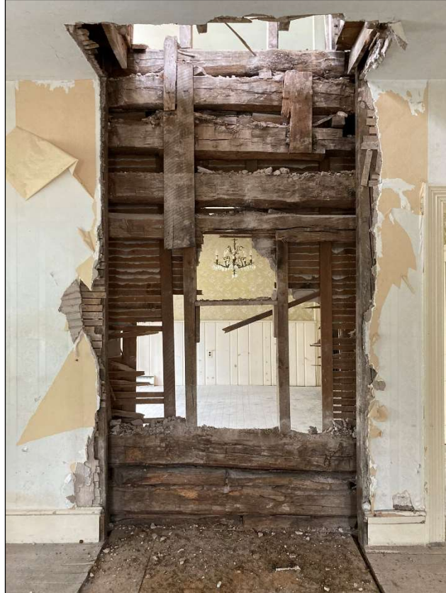
Figure 28. First floor, east front room, rear wall where chimney was removed. May 2023. Photo by the author.
