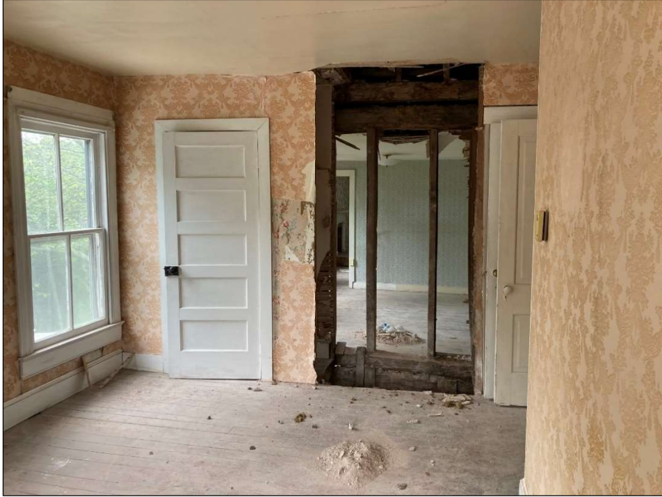
Figure 54. Second floor, east front room, looking at rear wall and removed chimney. May 2023. Photo by the author.
