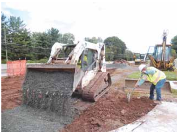
Workmen across from Rocky Run Middle School create what will be an asphalt bicycle-and-pedestrian trail along Stringfellow Road.
