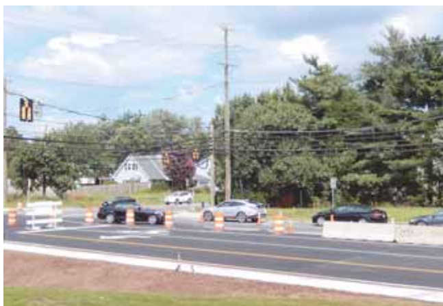
Southbound motorists are directed onto the old section of Stringfellow Road, while northbound traffic drives beside the new portion not yet open.
