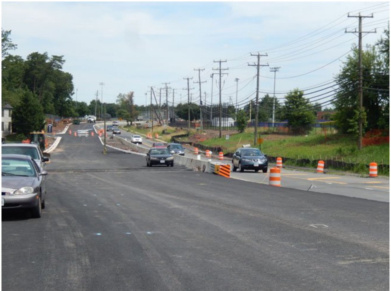
A newly asphalted section of the widened Stringfellow Road between Chantilly High and Rocky Run Middle School. Photo by Bonnie Hobbs .
